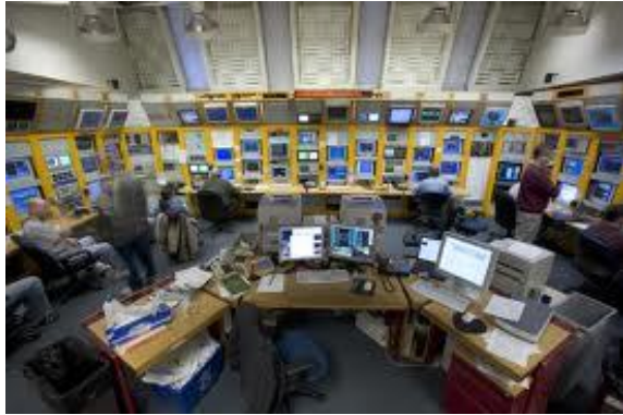
Tevatron's control room (USA)
