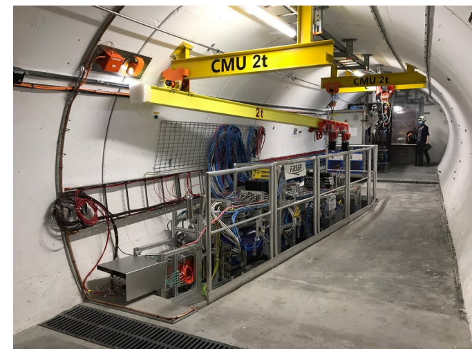
04/2021 FASER detectors in place
