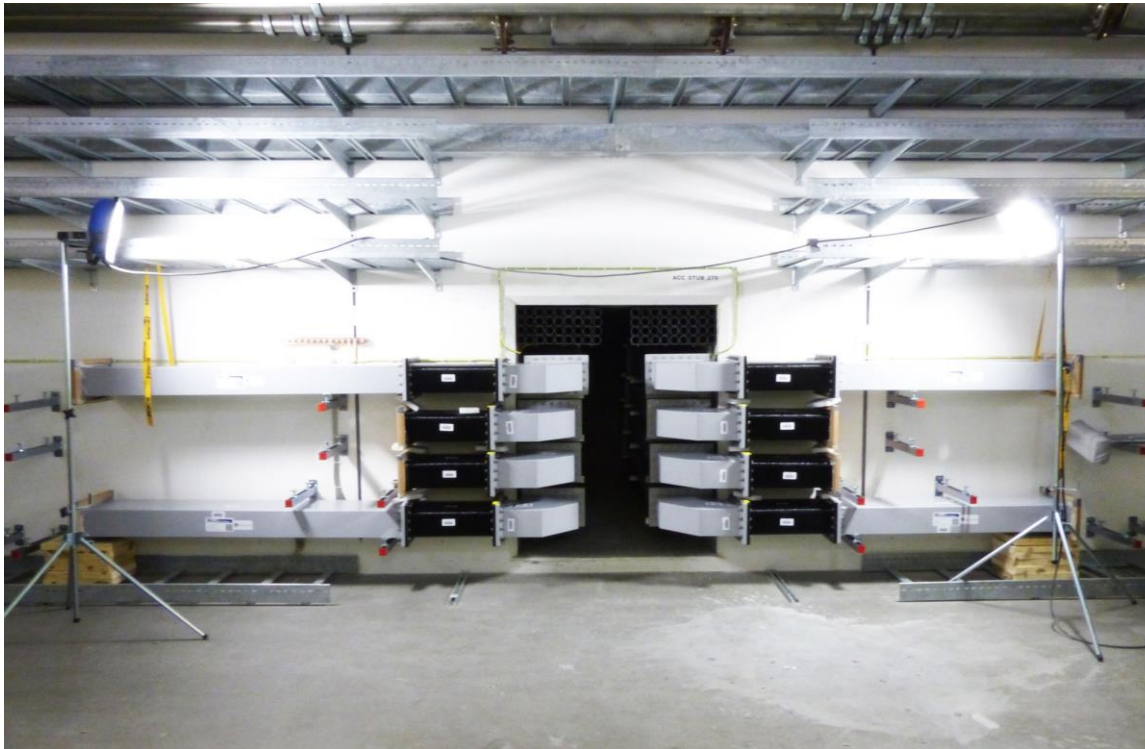
Waveguides installed in stubs. Many concerns (space, installation, etc.) but the end result looks quite neat.
