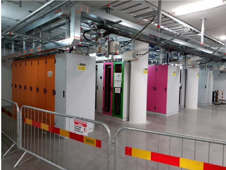
Equipment racks installed and populated
