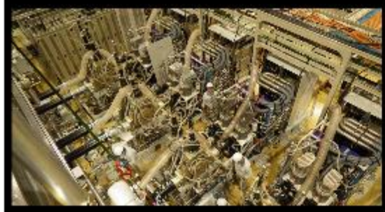
RF module for RFQ (Tetrode system) (INDRA, Spain) 175 MHz, 200 kW, CW × 8 chains
