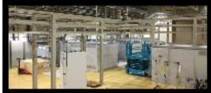
High Voltage Power Supply (HVPS) (JEMA, Spain) 13 kV, 400 kW × 8
