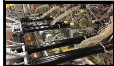
RF transmission line (Spinner, Germany) 9 8/16" Coaxial wave guide
