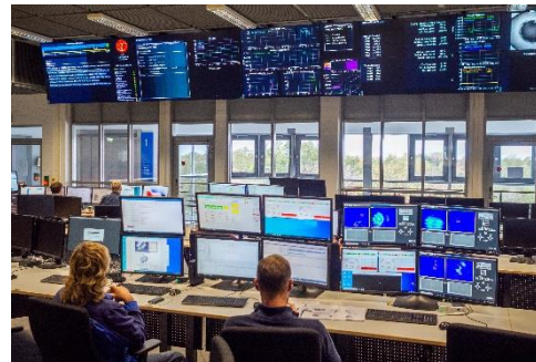
W7-X control room
