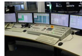
cSS operator workplace in W7-X control room
