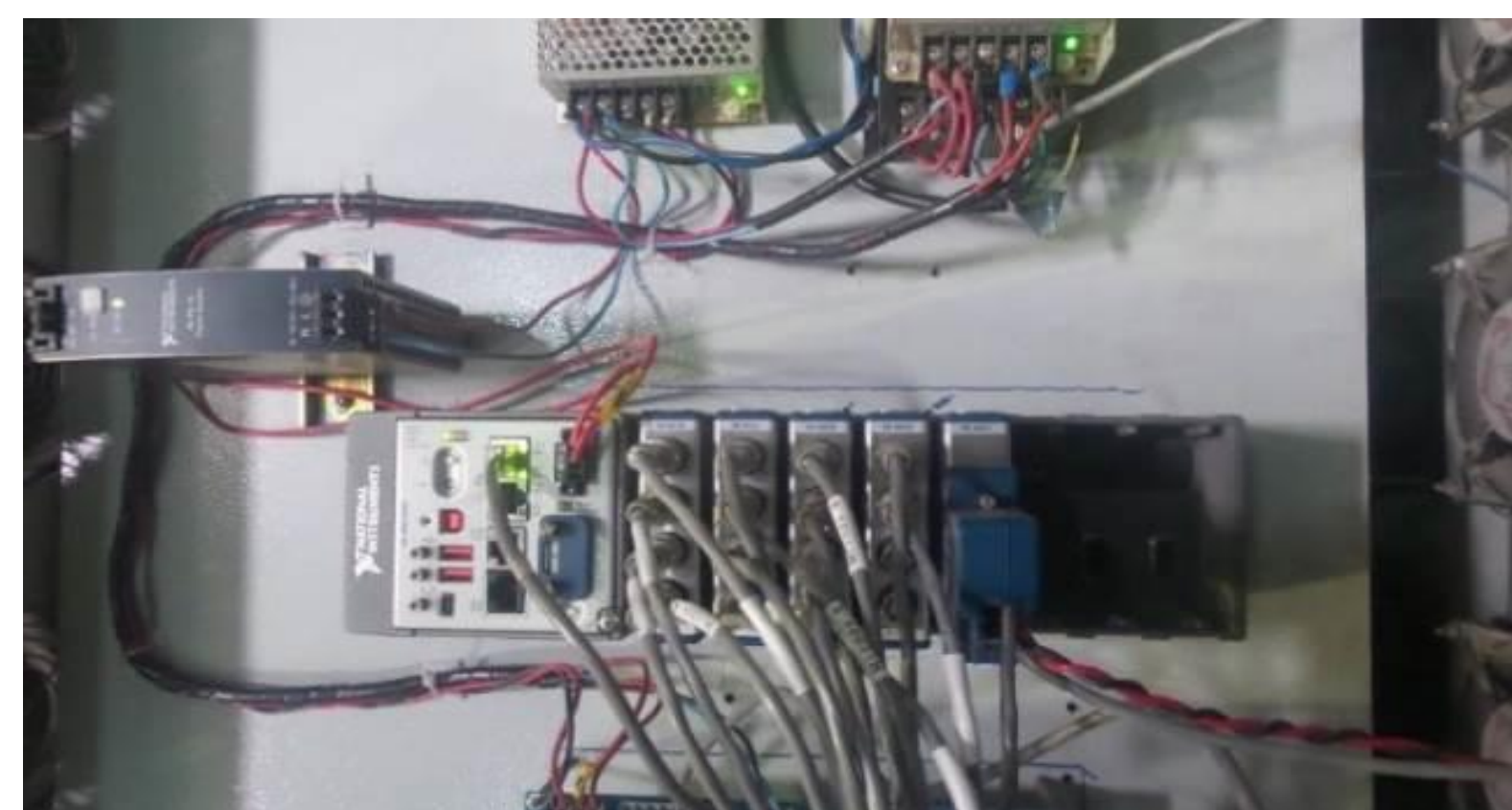
Installed cRIO platform
