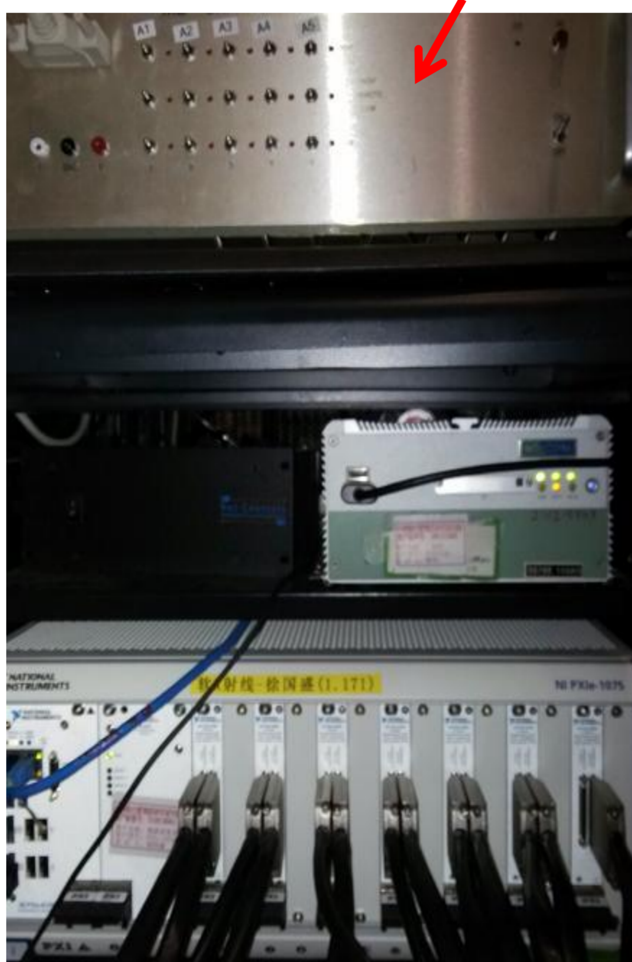
Gain controller: five electronics with 15 switches
