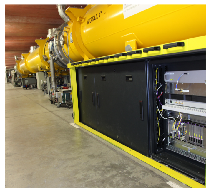
A MicroTCA.4 LLRF installation in the FLASH accelerator tunnel
