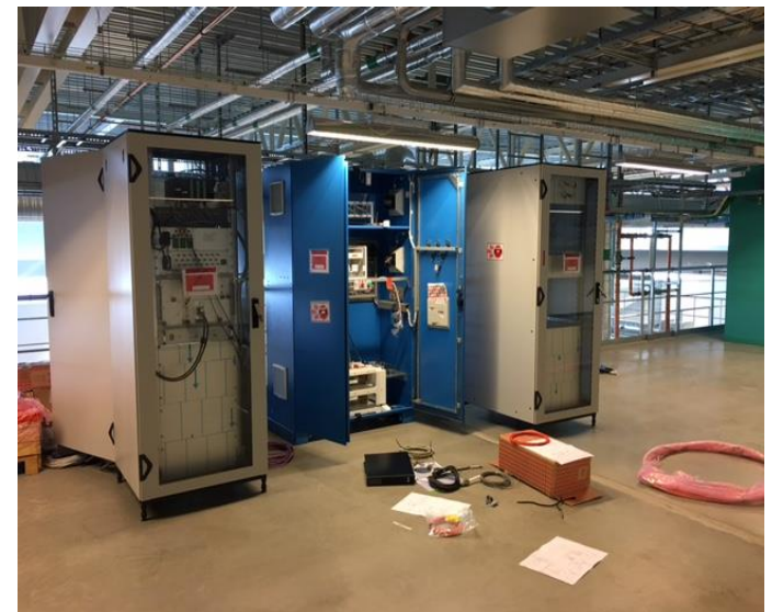
MIK pulsed power supply, control cabinets and high voltage charging power supplies at MAX-IV.
