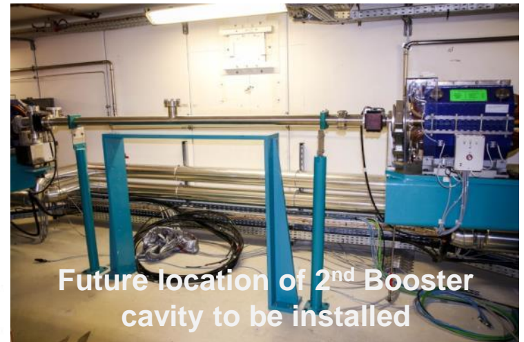
Only the cavity is missing
