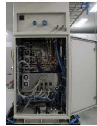
LCLS-II: 3.8 kW 1.3 GHz (284 units)
