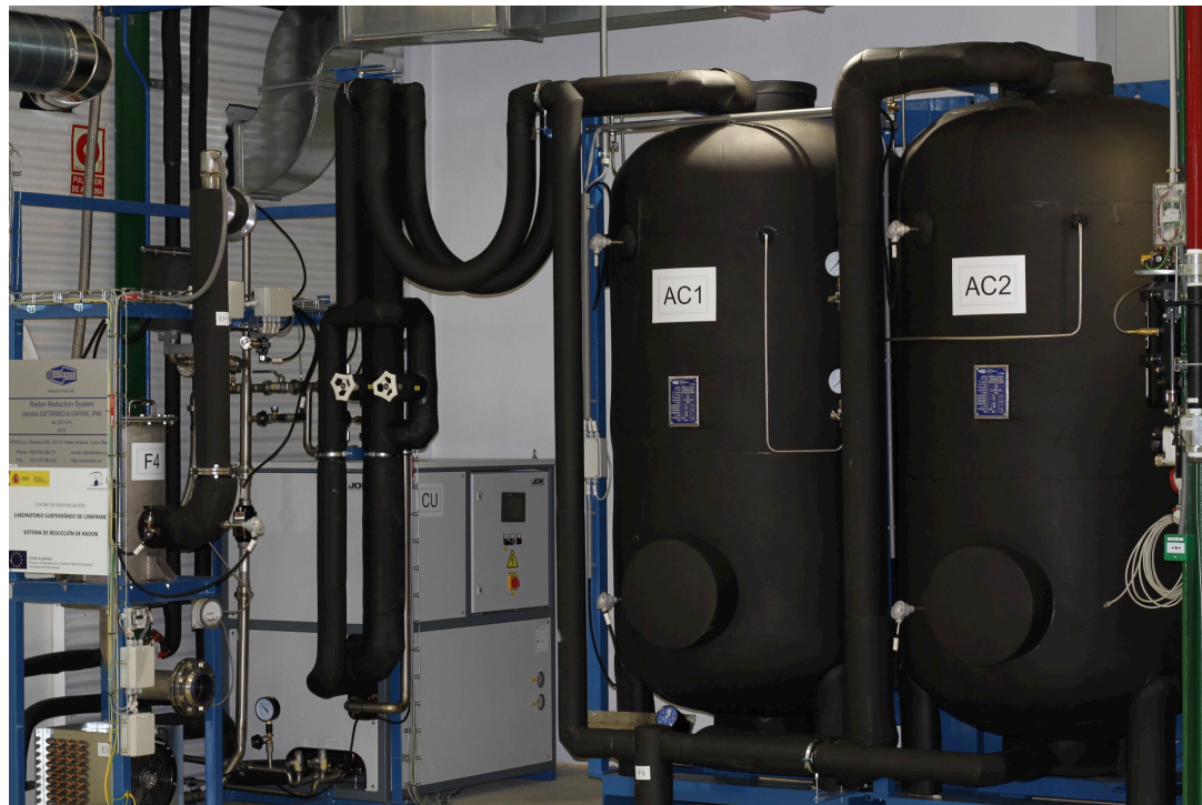
Radon abatement plant
