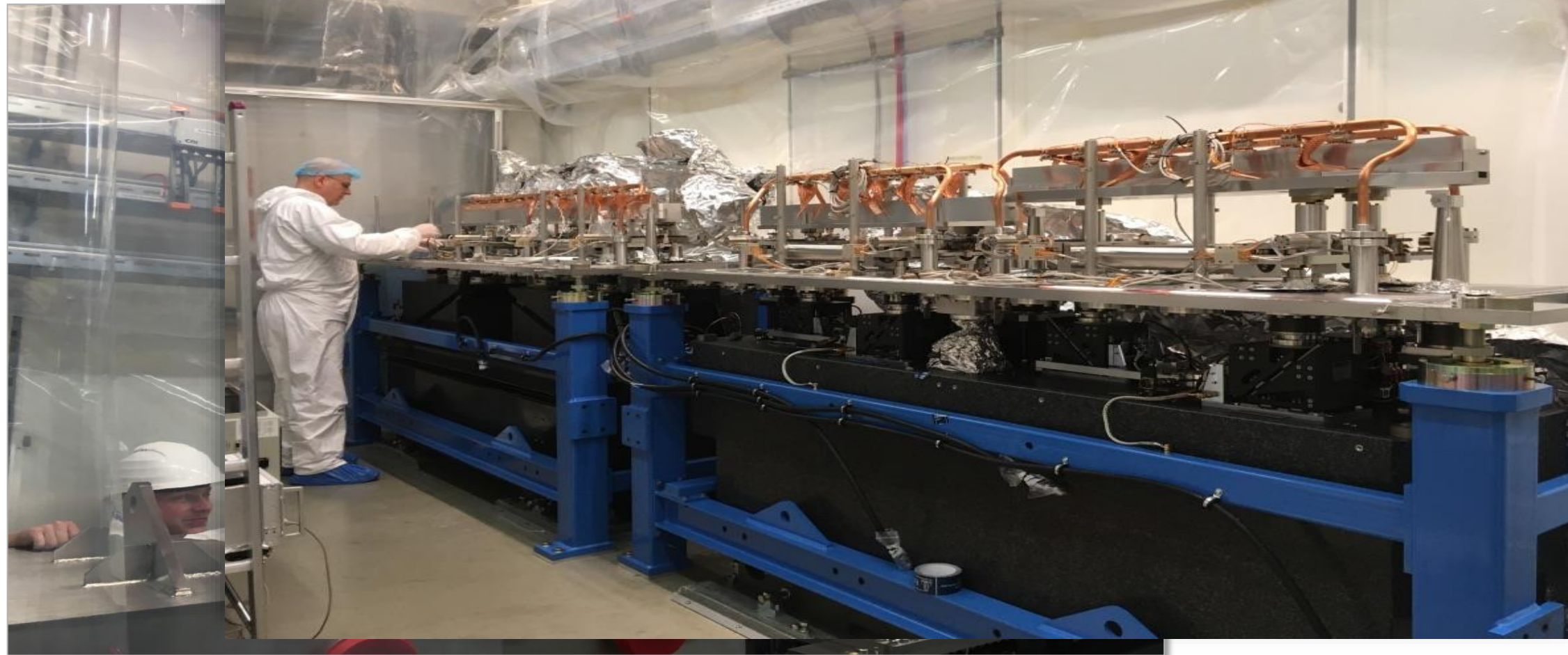
Optics hutch installations (mirror chambers) in early March
