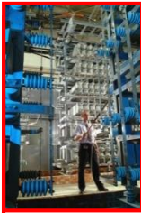
Main magnet capacitor bank
