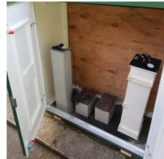
Roadside cabinet inside
