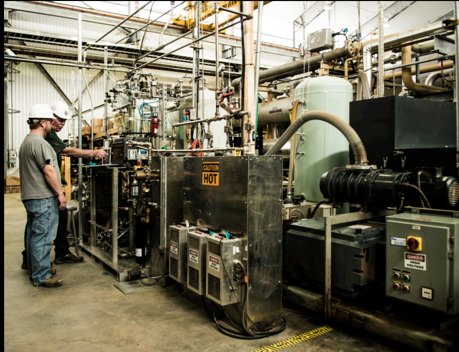
Plant at Colorado
