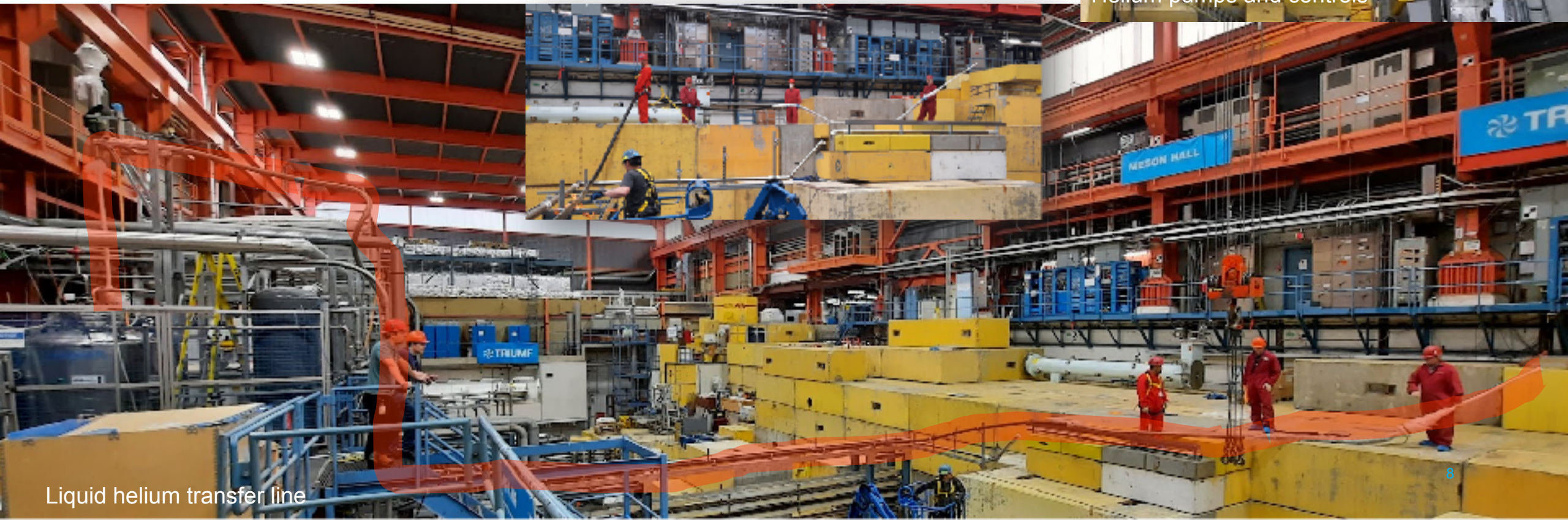
Helium pumps and controls
