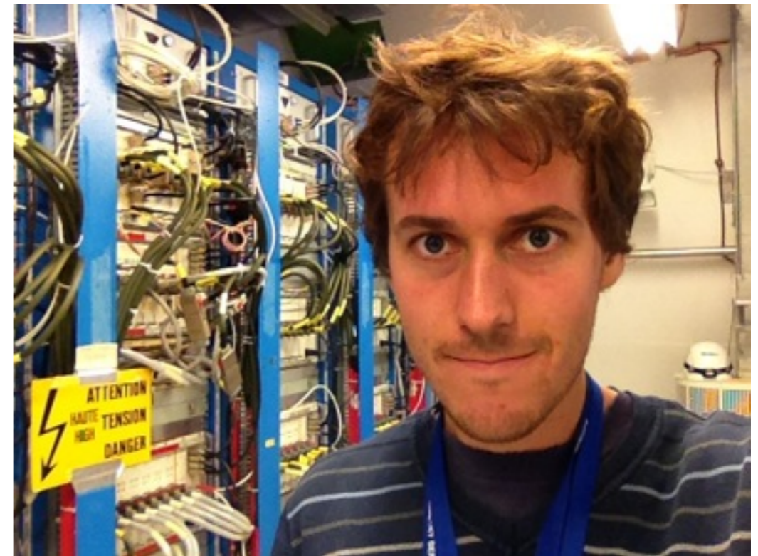
Canadian graduate student at work in ATLAS underground in Fall 2013 - LAr HV System in counting room (*he put on his helmet after)
