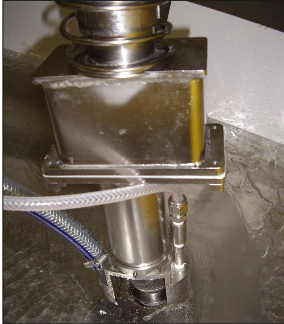
UPW flushing and Acrylic/UPW extraction lines
