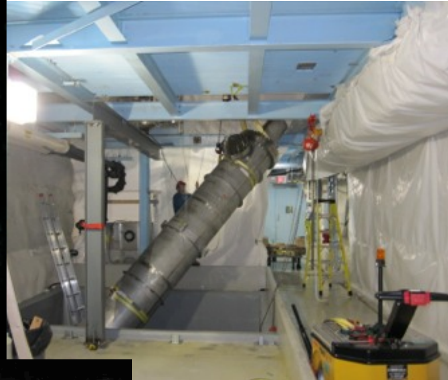
First LAB plant vessel being installed into utility drift (prior to completion of steelwork)
