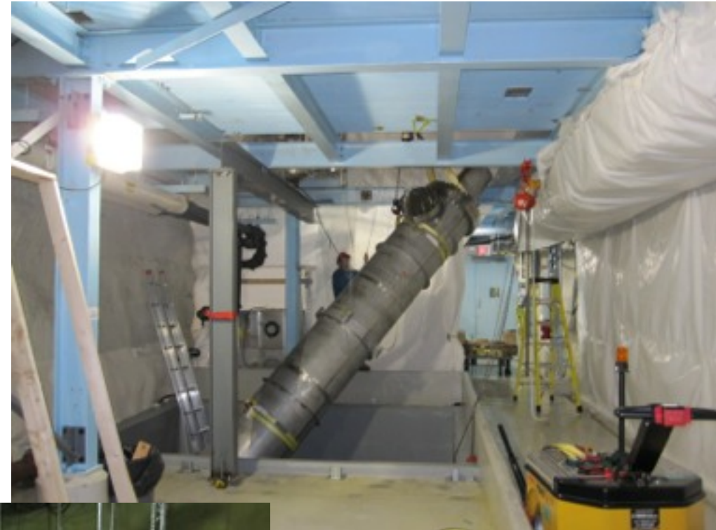
First LAB plant vessel being installed into utility drift (prior to completion of steelwork)
