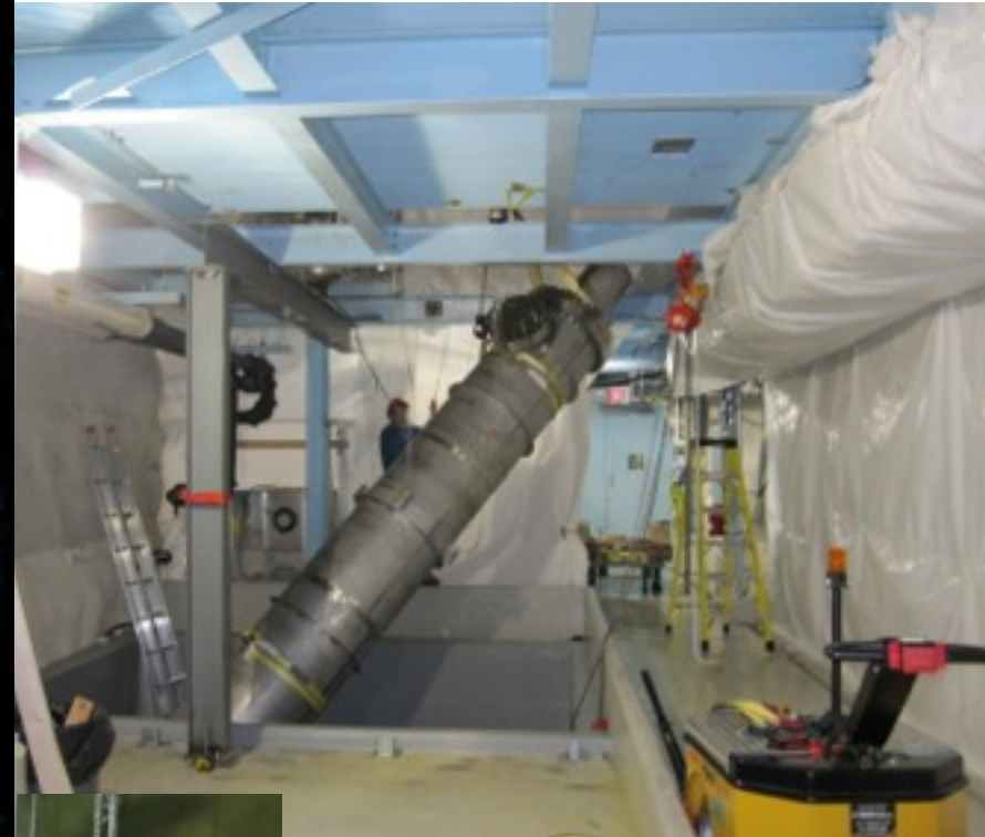
First LAB plant vessel being installed into utility drift (prior to completion of steelwork)
