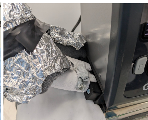
Chiller leak and frost
