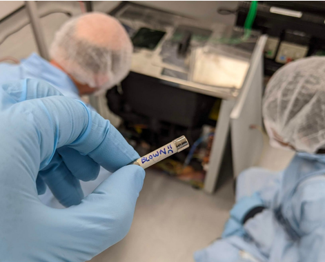
Blown chiller fuse
