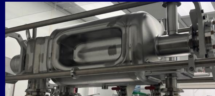
NRPD04 being assembled at ANL
