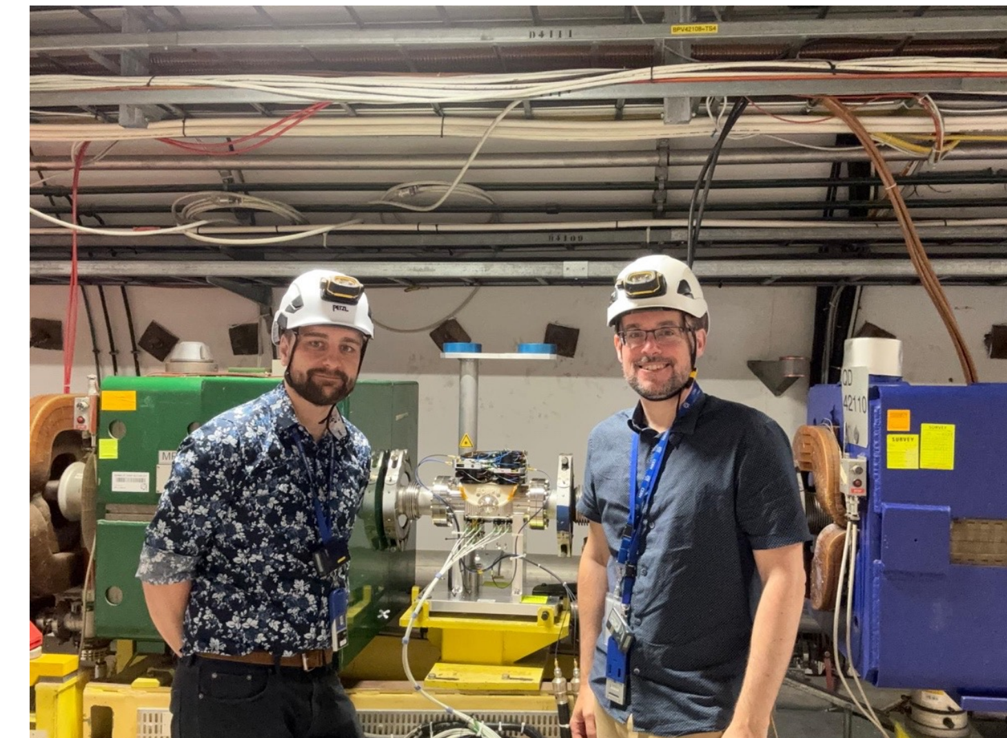
June 2025 installation of new adjustable EO pickups
