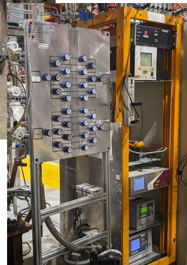
Inline filters and gas analyzer system
