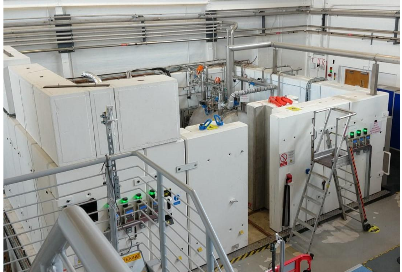
High power testing with LHe – including cleanroom & HPR infrastructure
