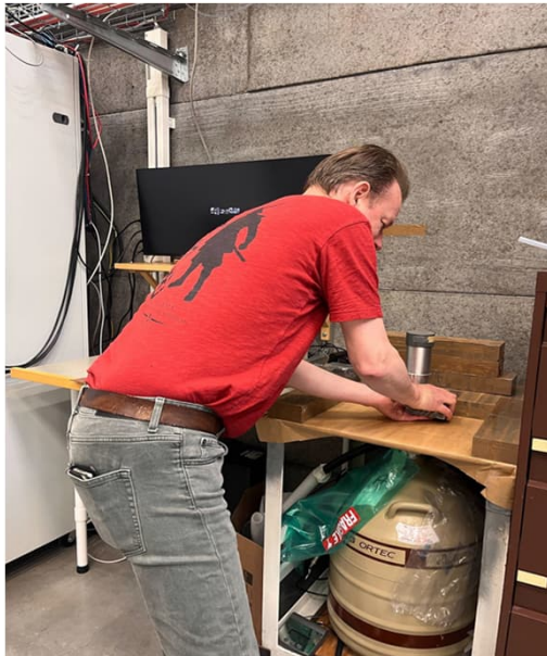
Building up the lead castle for HPGe in NESSA
