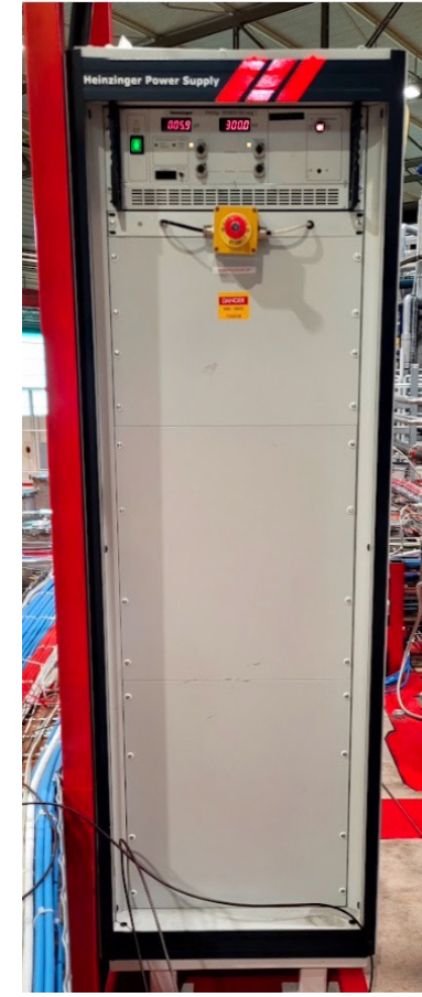
HV power supply
