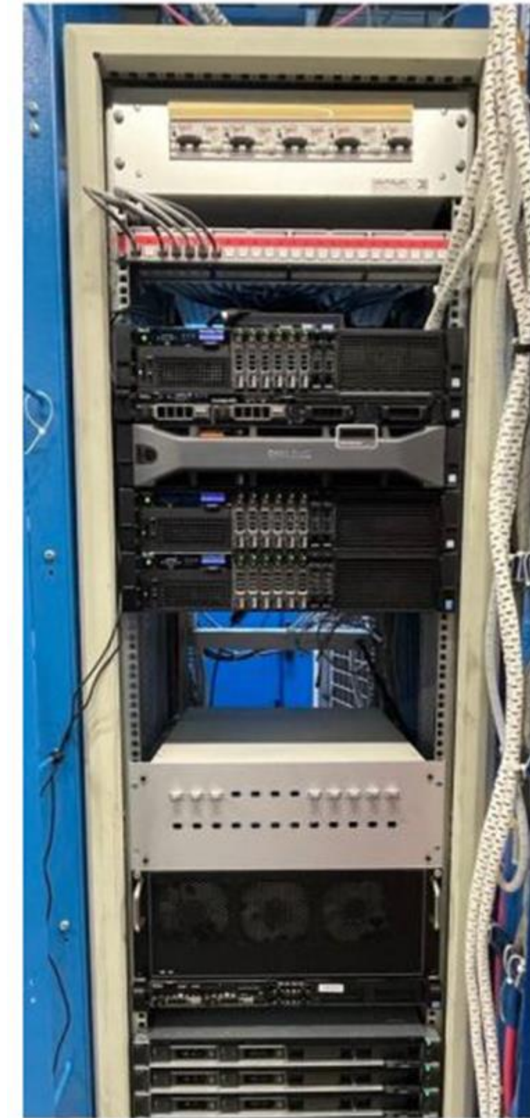
Level-1 Data Scouting rack
