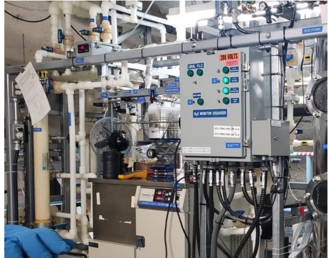
UPW plant Radon board, 2026
