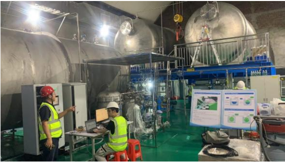
Filling Overflow Circulating room
