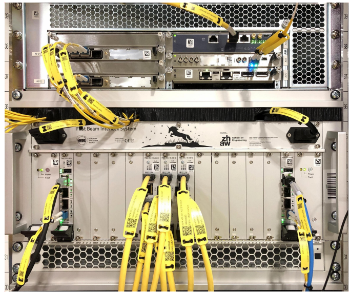
Fig. 2. DLN crate (top, mTCA 3U) and SCU crate (bottom, cPCI). In the DLN, the two IFC1410 boards implementing the interlock logic are on the left; the MCH, EVR, and Concurrent CPU are on the right; yellow fibers on the IFC1410 front panels are the incoming Slinks from the SCUs. In the SCU, the two Serializers are at each end; the three RS485 MCs at the centre connect to five BLMs via discrete RS485 signals and Ethernet datalinks; yellow fibers exiting from the bottom of each Serializer are the Slinks to the DLN above.
