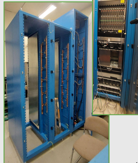
CERN - SRI Main location for integration tests
