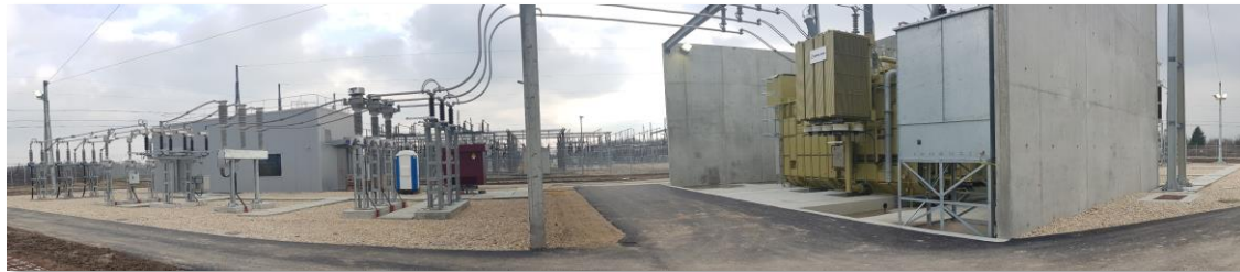
New 400/66kV BE2 sub-station
