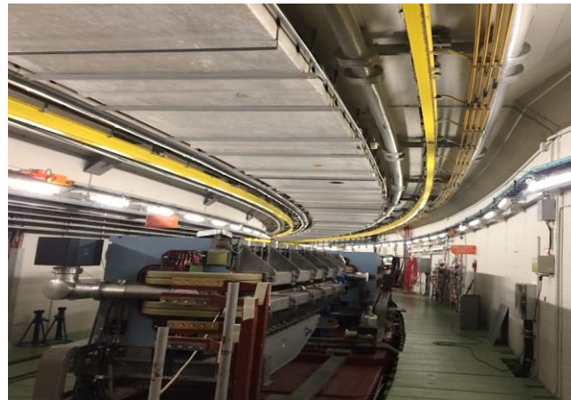
Electrical infrastructure in injectors consolidated during LS2
